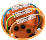
Wiring conductors in a flush-mounted junction box.
